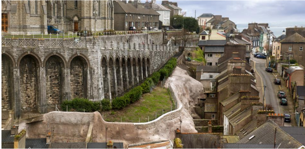
Figure 2. 3 Shotcrete protection on a slope at Saint Colman's Cathedral, previously at risk (3)
