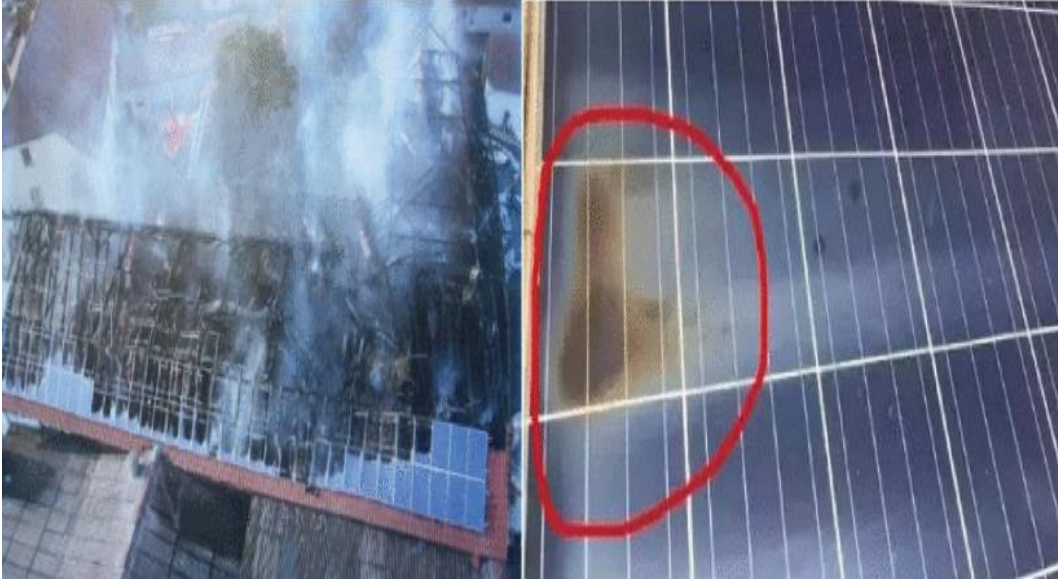
Figure 1.4 Fire incident in PV array initiated by hotspot failure [46].
