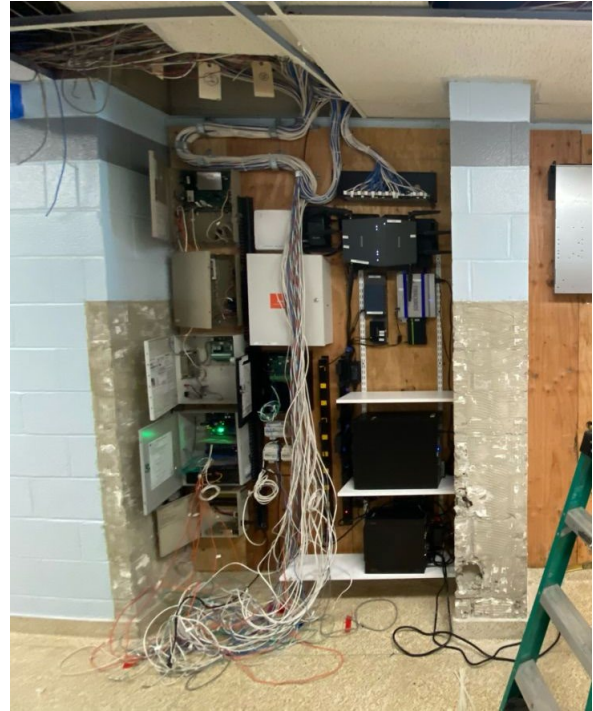
Figure 22 — (a) Employee Opens Office Door with Badge [6] ; (b) Access Control Installation in a Public Building in NYC [7] showing cables required
