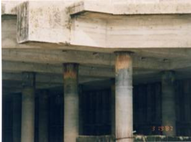
Figure 1. Steel piles with Corrosion.
