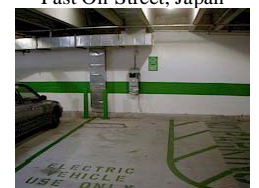
US Disabilities Compliance EV Parking Bay in a MSCP
