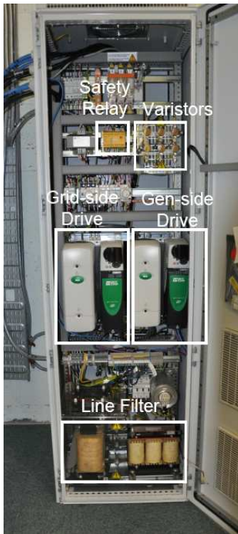
Figure 8 Regenerative Drive Panel
