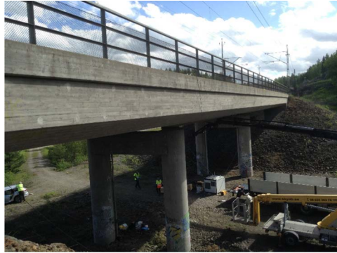
Fig. 2. Photograph of Pershagen Bridge, Sweden used for testing a deployment of energy harvesters.
