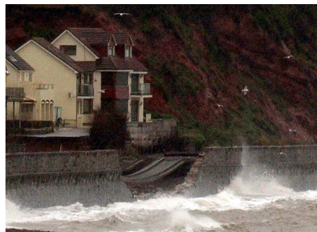
Figure 3: Seawall collapsed at Dawlish on 6 February 2014, with rails hanging in mid-air. Source: http://www.geograph.org.uk/photo/3838795 . Copyright: Derek Harper, Creative Commons Licence.
