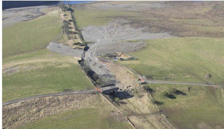
Figure 11.5 Camerton bridge collapse (Photo credit: Simon Ledingham).
