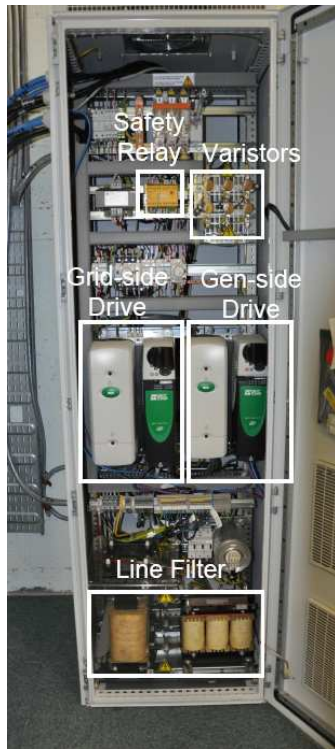
Figure 8 Regenerative Drive Panel
