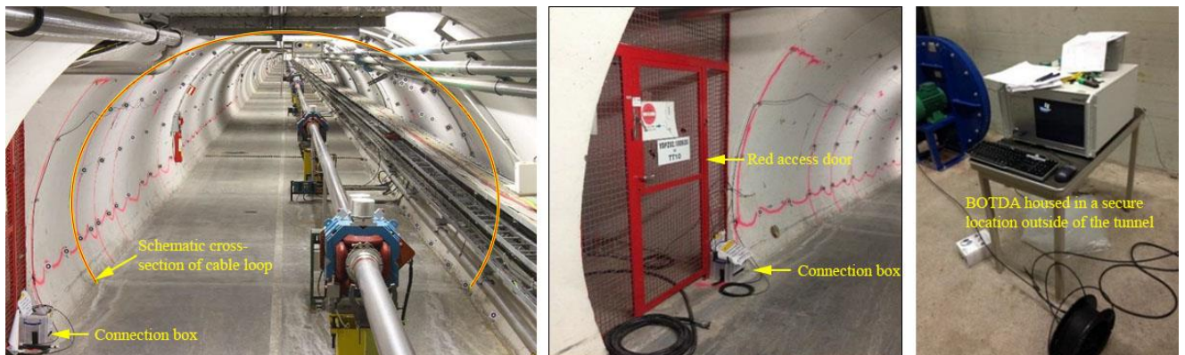
(d) DFOS onsite deployment, cable connection box and BOTDA
