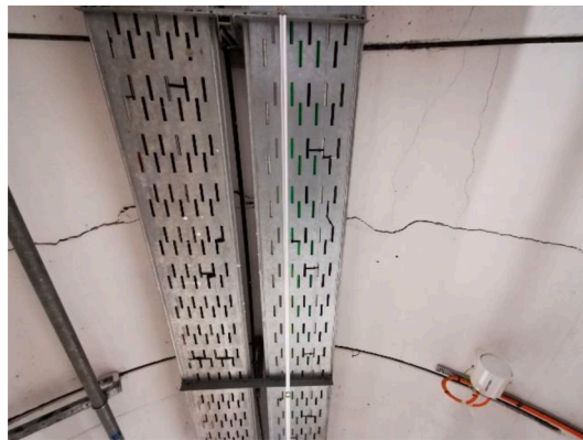
(a) circumferential cracks along cross section
