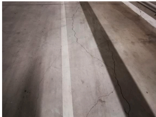
(c) longitudinal cracks at tunnel floor
