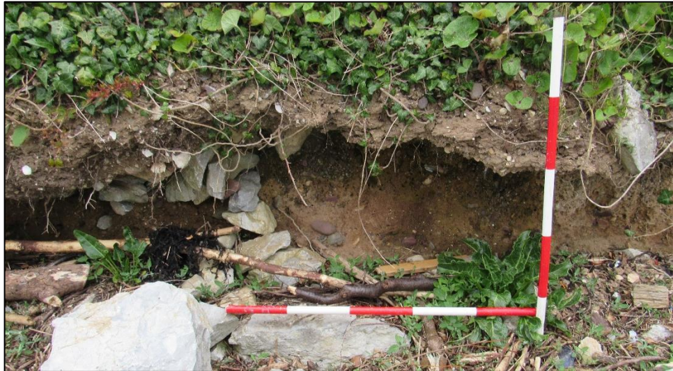
Figure CO.2: 1 square metre sample of section showing undercutting.
