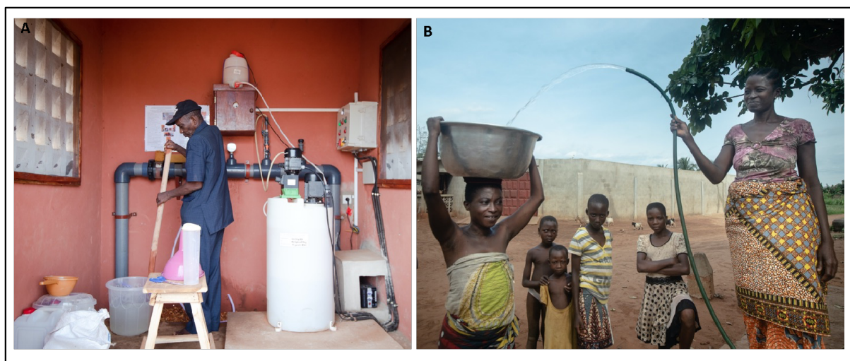
Figure 26. Chlorination system in water tank station (A) and water fountain (B). Photo taken by Odilon Amour. Benin, 2020.
