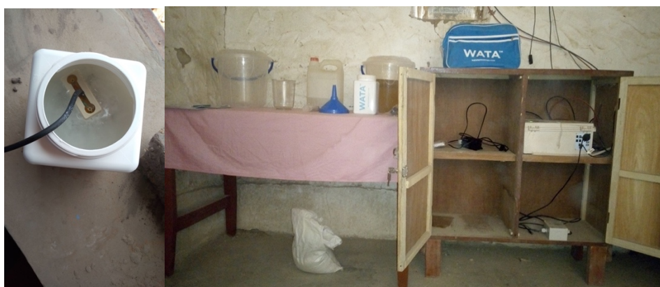
Figure 23. Photo of an electro-chlorinator device and a production room.
