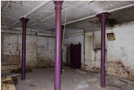
Plate 7.17 Engine room at the Belfast and Ulster Brewery. Note the brick-built, triple jack arched ceiling supported on cast-iron columns and the sliding fire doors.
