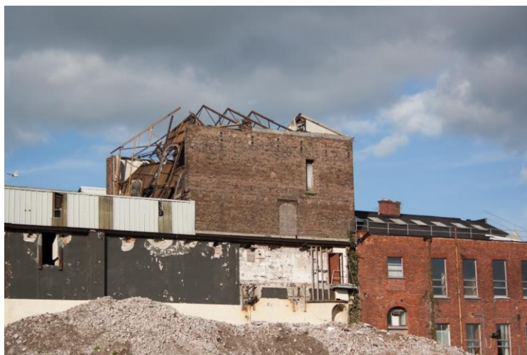
Plate 5.4. Malt-milling loft at Beamish and Crawford following damage received in hurricane-force storms in October 2017.
