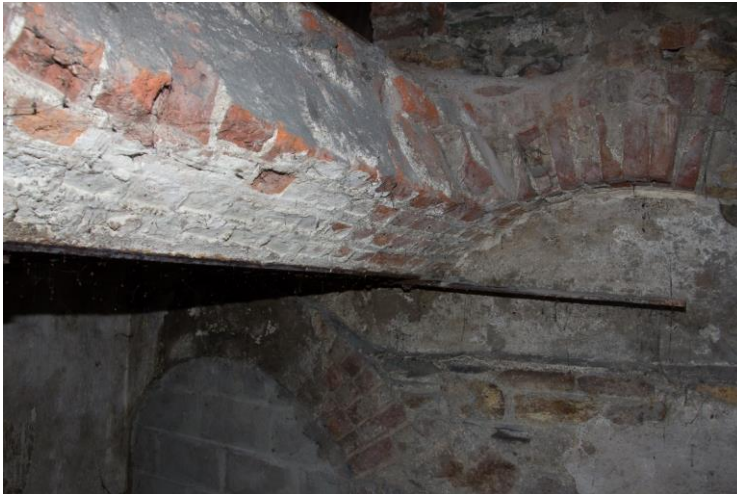
Plate 5.20. Remains of barrel-vaulted furnace arches, the Mill Park Brewery, Enniscorthy.
