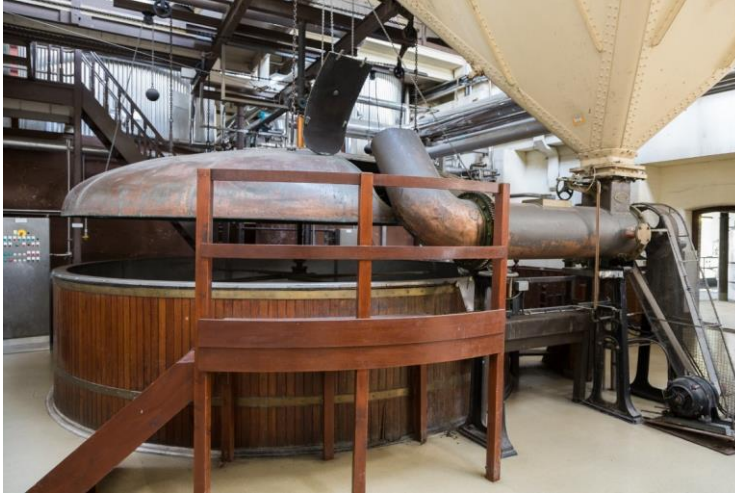
Plate 5.7. Steel's mashing machine with cast-iron grist case, belt-driven by an extant electric motor. Mash tun no. 3, the St. Mary's Brewery, Waterford.
