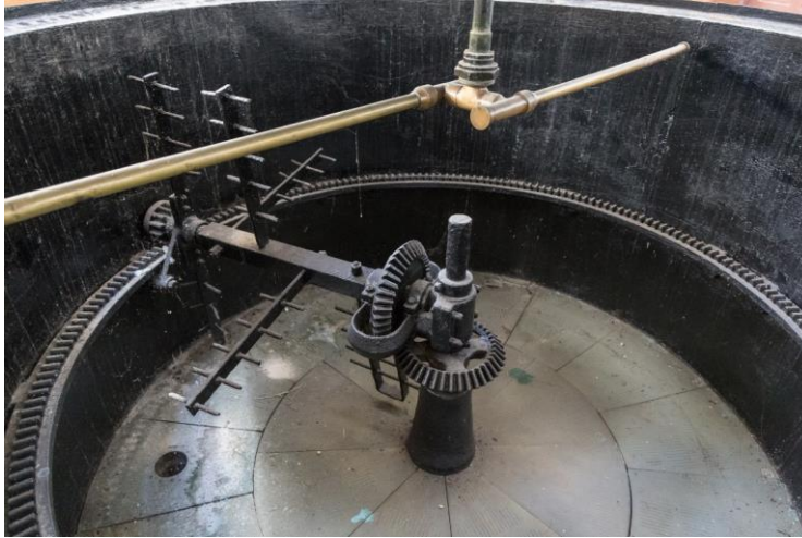
Plate 5.6. Interior view of mash tun no. 1, the St. Mary's Brewery, Waterford. Note the perforated base plates, mechanical mash rakes and sparging mechanism suspended from above.
