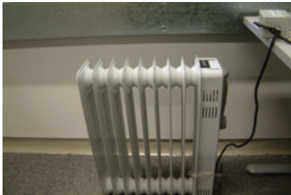
Figure 9: Wireless actuation for heat radiators
