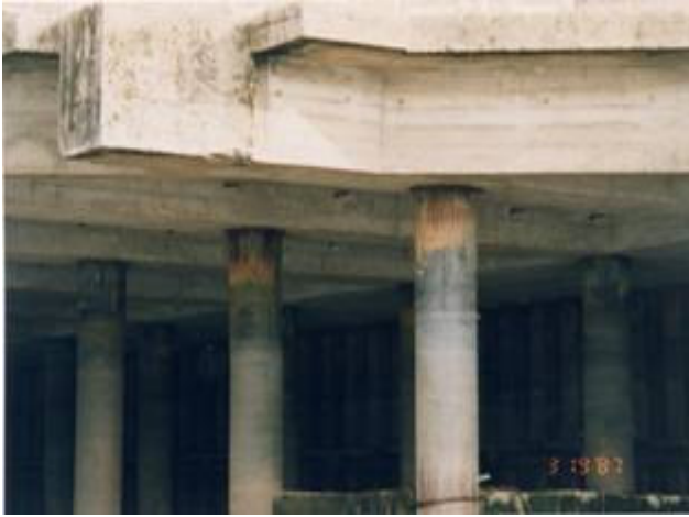
Figure 1. Steel piles with Corrosion.
