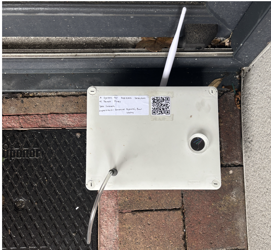
Figure 4.2: LoRa Dragino sensor node 1 setup in a test environment
