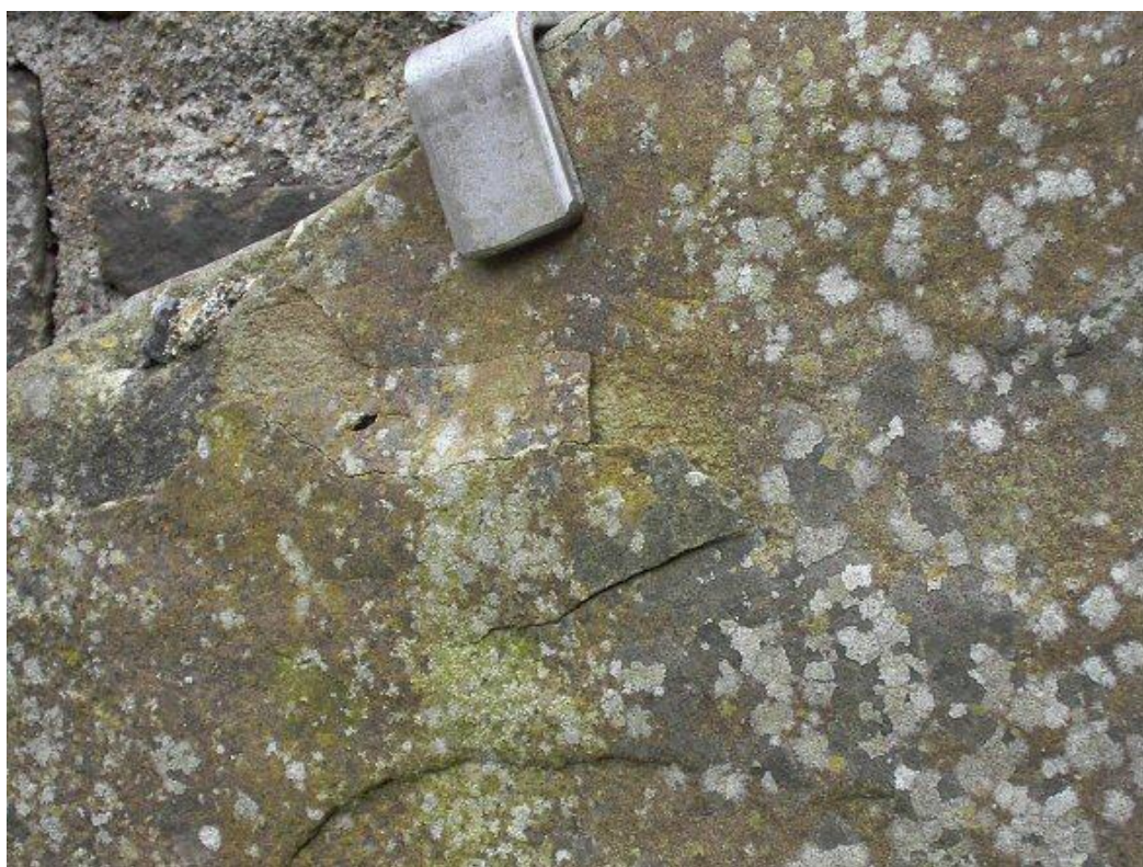
Image 45: Tullylease, image showing flaking of sandstone
