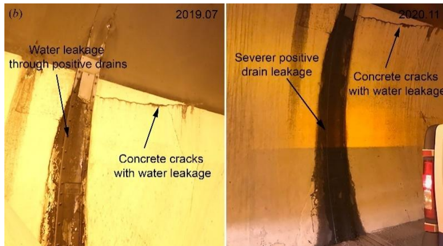
(1) Tunnel surface defects at UAV inspection area [216]
