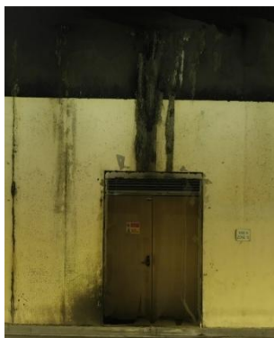
(1) From lining cracks
