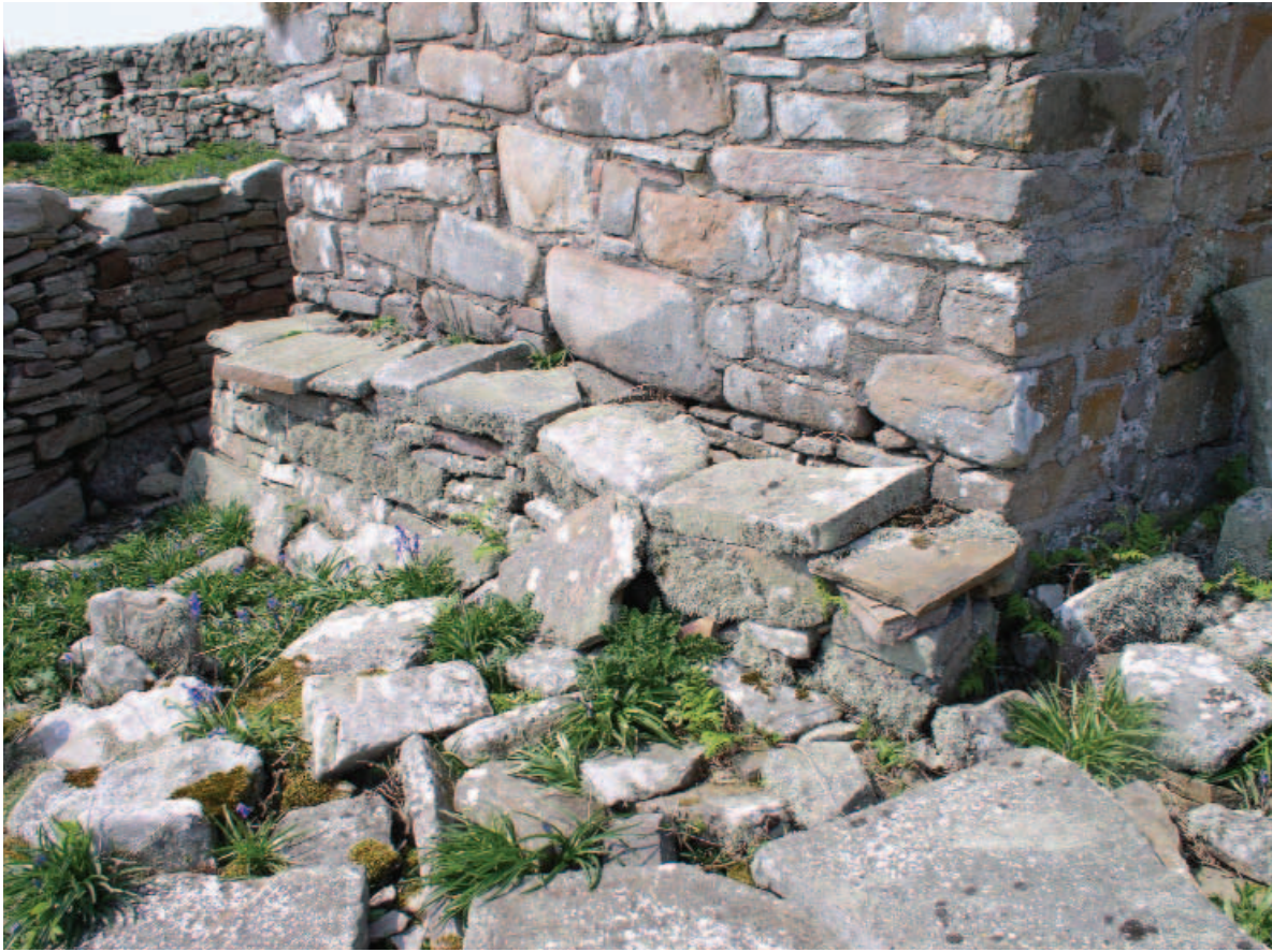
Plate 24 Fragile medieval buildings are vulnerable to damage by visitors as well as the elements: unstable wall bench on the south face of Teach Molaise.
