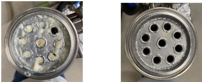
Figure 5: Top down view of the inside of the shell and tube heat exchanger, showing the heat exchanger fouled (left) and unfouled (right).
