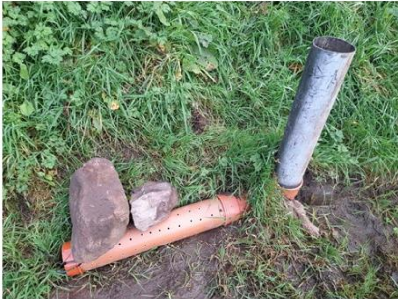
Figure S1B1Top: DB outlet pipes in lowered position to allow fast draining stored water from the DB. Bottom: Outlet pipes amended 1 st Nov 2021. Left pipe was capped and perforated along its length to allow slow, constant drainage of stored water; right pipe is secured in upright position to allow fast draining of water once the DB reaches a maximum depth of 0.85m above the topographic minimum
