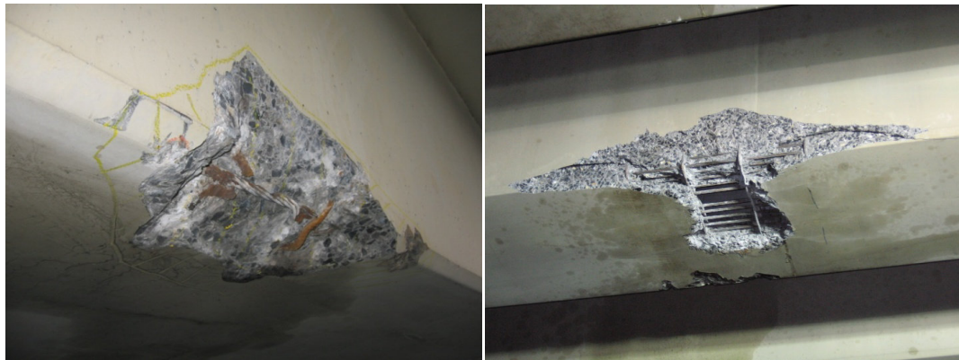
Figure 6.1 Damaged region of outer beam (left) and inner beam (right) [190].
