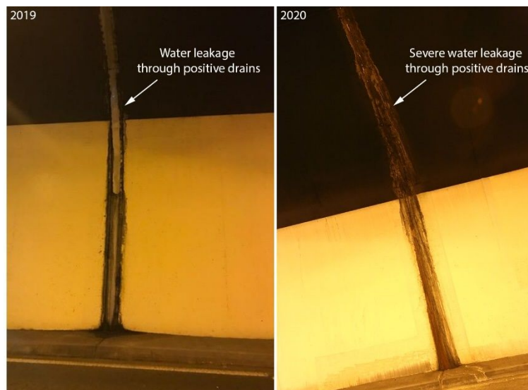
Figure 3. Progressive tunnel lining deteriorations at VCP 16 section
