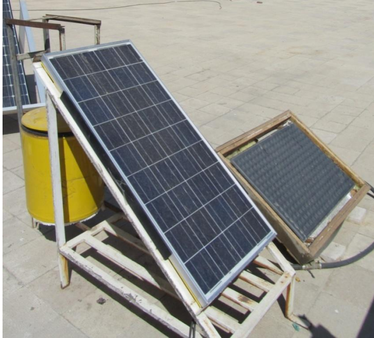
Figure.3. PV/T collector system
