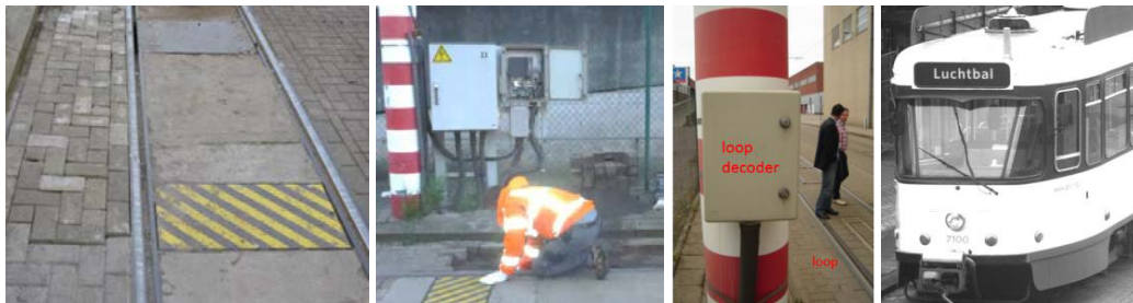
Fig. 6. Wayside axle bearing monitoring system for Light Rail Vehicle.
