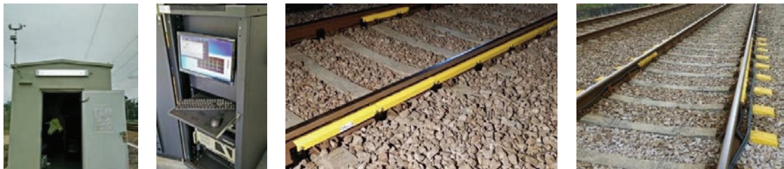
Fig. 4. Wayside system in Portugal: data processor unit and system installation in the track.
