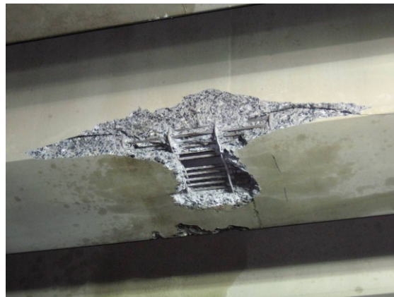
Figure 2 – Photograph of Impact Damage
